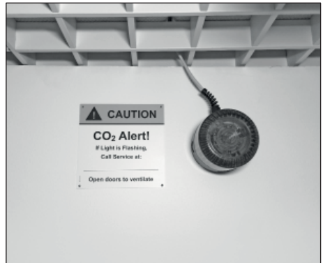
Warning lamp with sign
