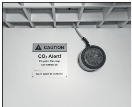
Warning lamp with sign
